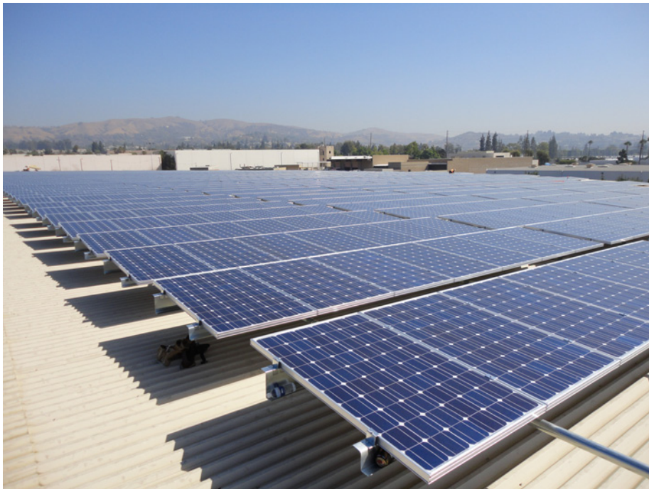
Power generated by the solar panel arrays atop the reservoir at the Maintenance Yard will help to mitigate future water pumping costs.
