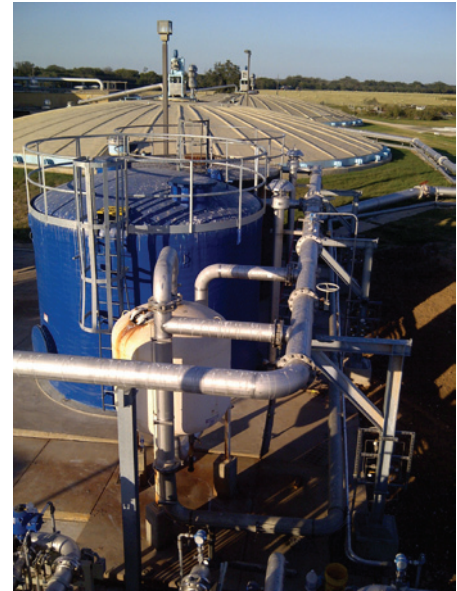
The combined heat and power system at the Hornsby Bend facility will offset current plant electrical consumption and support heat demands of the anaerobic digesters, which in turn produce biogas fuel for the generator.
